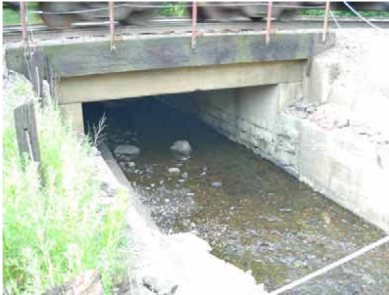
Looking at double box culvert that contains flow of Indian Creek, at the west end of the Eola yard, west of Farnsworth Ave.
