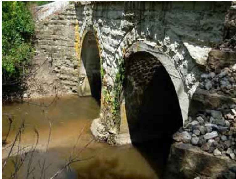
5. Looking west at the double arched culverts open bottom culverts within the IAIS rail embankment
