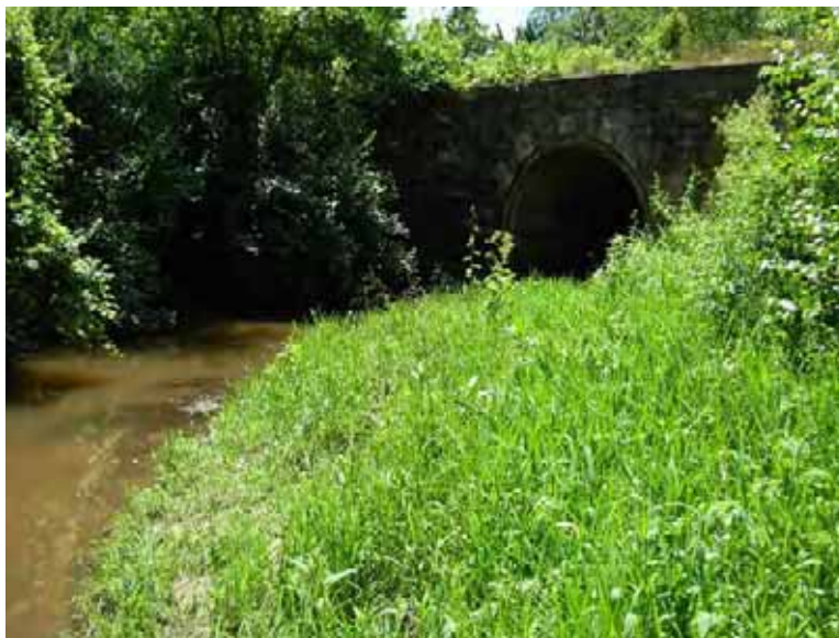
6. Looking south toward the IAIS railroad from within the Pond Creek floodplain
